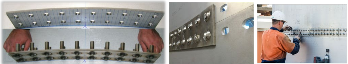
Figure 9 – Albion Leach Reactor-Lap Join System
