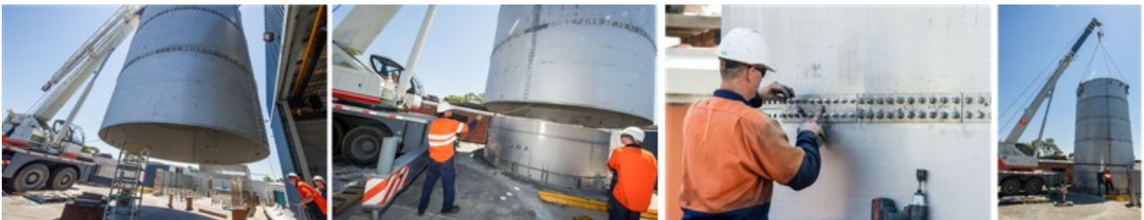
Figure 19 – Albion Leach Reactor Assembly
